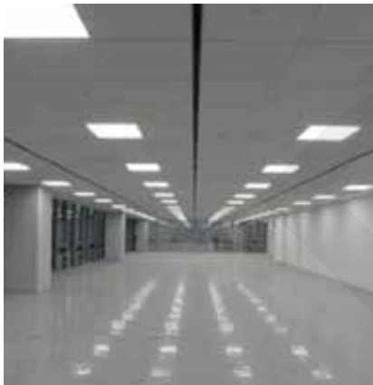
Highly efficient LED lighting
