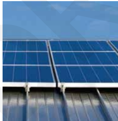
Roof mounted photovoltaic (PV) arrays
