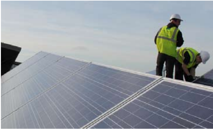
On the Slough Trading Estate, we signed an agreement with an occupier, AZUR Solar, to install 189 sq m of photovoltaic panels. These are expected to generate 22,000 kWh of clean power per year, enough to run three average homes for a year, saving 14 tonnes of carbon emissions.
