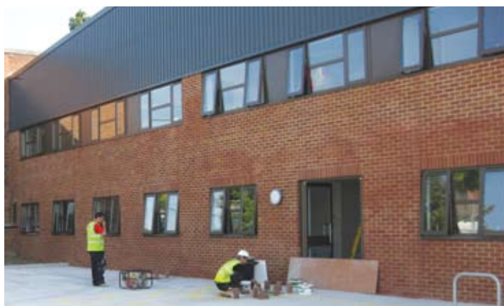
During our reconstruction of Abbeydale Road in Wembley, we used a steel framework and cladding system understood to be the world's first carbon neutral building envelope, with high levels of recycled content. The system's end of life performance is also strong, with 84 per cent reusable or recyclable steel content and 100 per cent recyclable composite steel panels.
